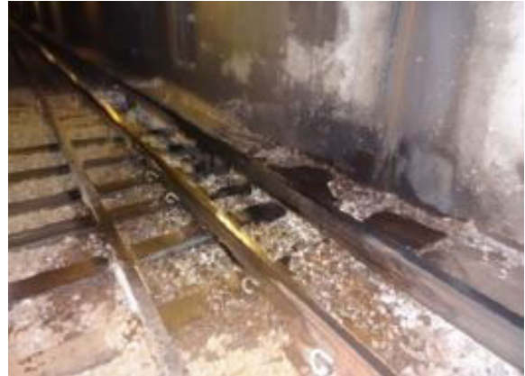
Existing Water Damaged Area at the Kimball Subway.
