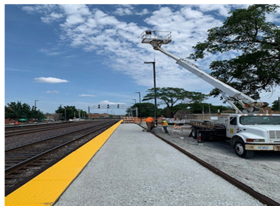
Workers install light fixtures at Melrose Park Station on the UP-West line.
